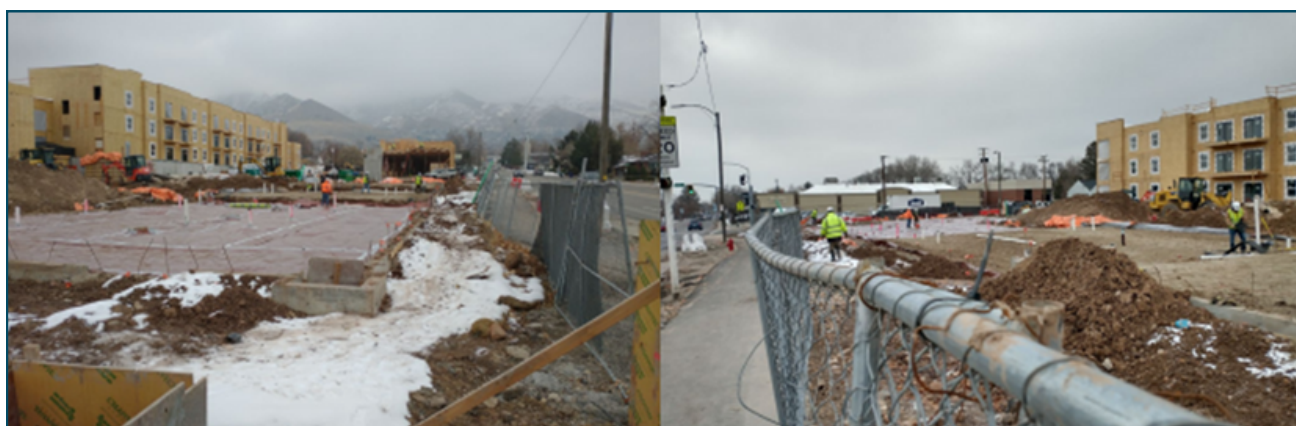
Installation of the vapor intrusion mitigation system at the 21st and 21st Site, the Former Blue Plate Diner (Photo by Dale Urban)
